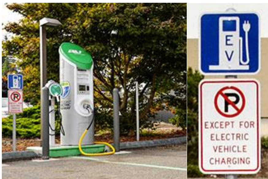
Figure 15. PEV signage and green pavement lines required in Washington, Oregon and California 87
